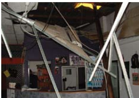
Surveying the damage and tarping the hole in the roof
