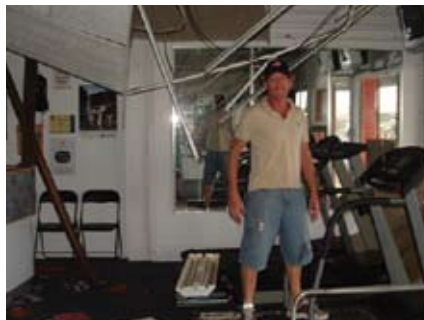
Surveying the damage to the ceiling
